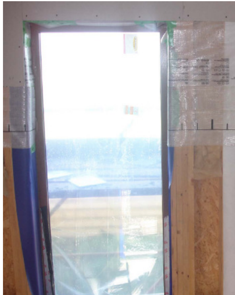
Sealing under way at junction of timber frame wall and external wall ope
